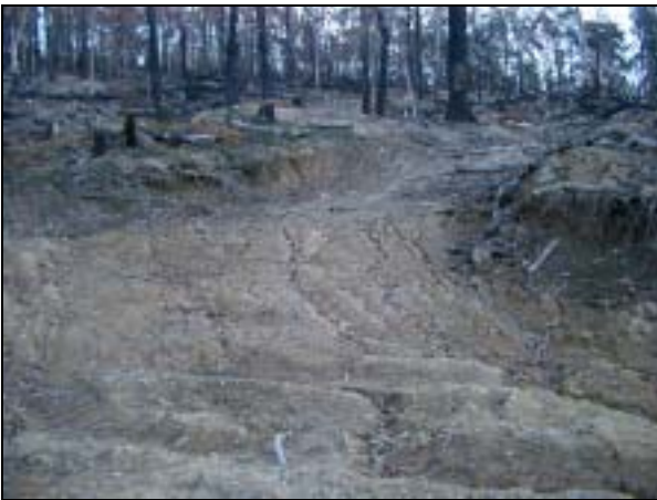
Photo 8. An example of erosion on an internal road.
