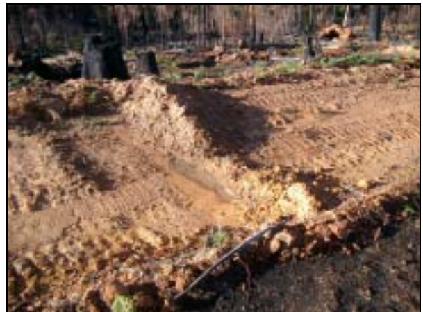
Photo 24. An ineffectual cross-drain. The bar is perpendicular to the road alignment and slopes back from the breach visible in the upper section of the photograph.
