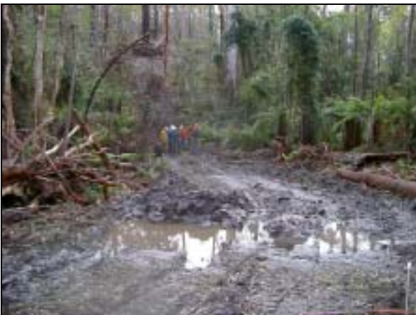
Photo 21. Boundary track installed through filter strip by DSE after completion of harvesting.
