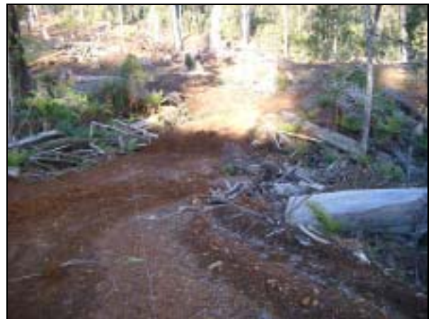
Photo 12. Track installed across filter strip by DSE without approval.
