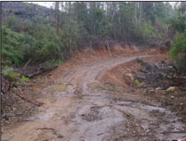
Photo 2. Section of the permanent road shown in Photo 1 constructed without table drain and proper cross-slope or crown.
