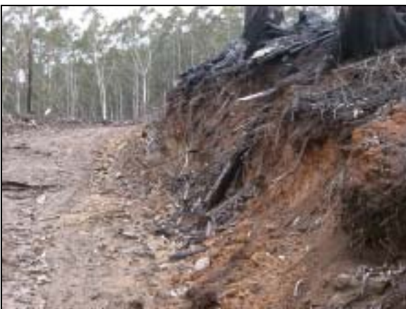
Photo 15. Roadside batter finding its own angle of repose.
