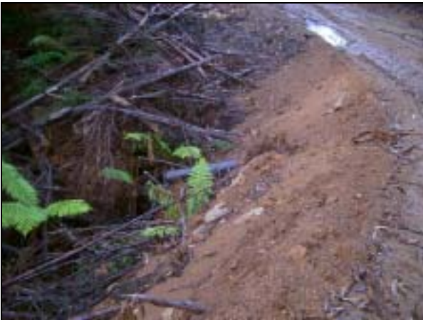
Photo 1. Steep fill batter installed next to road with undersized culvert.
