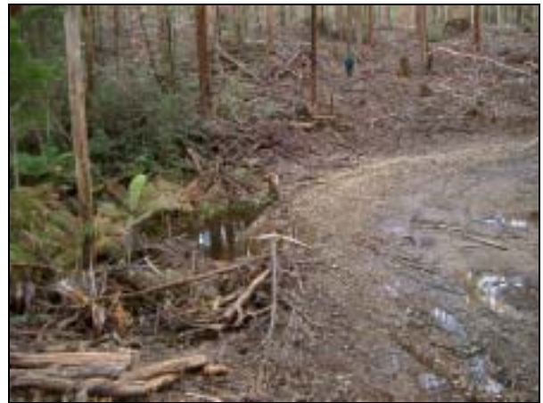
Photo 17. Road culvert blocked by damage from excavator. Note water running across road.
