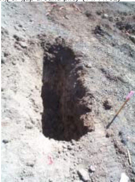
58. Test pits used to sample soil along eastern boundary of site (near location of burial of contaminated soil on-site) (14/11/02)
