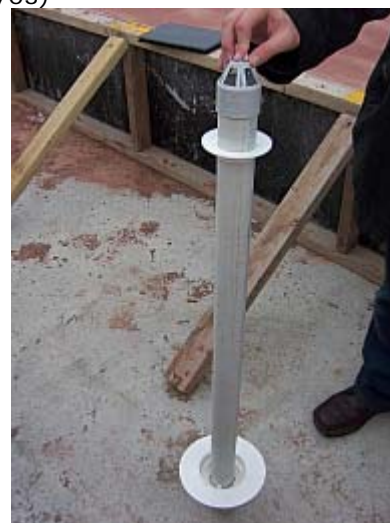
73. Gas vent assembly (17/6/03)
