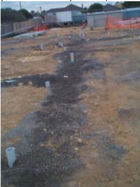
52. Services installed in trenches beneath supermarket where cap was locally thickened (28/10/02)
