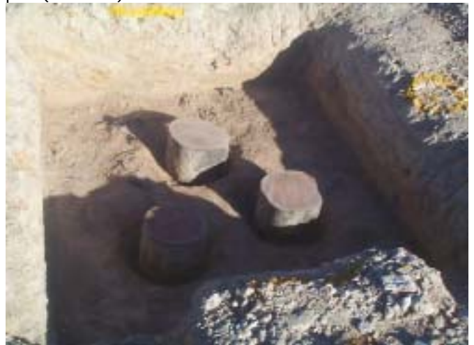
44. Excavation for construction of pile cap (note cracking and gap around pile reduced after excavation – ie cracking appears surficial) (25/9/02)
