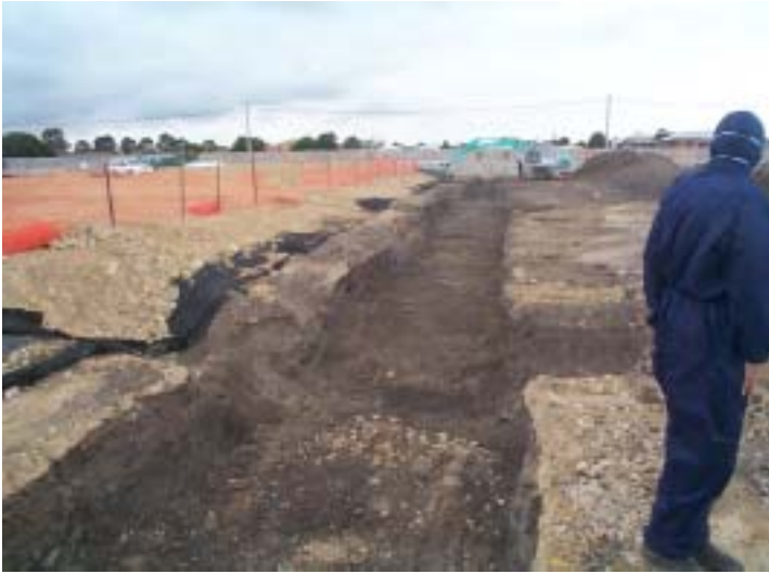
50. Excavation of service trenches (for placement of clay) in eastern portion of the site (28/10/02)
