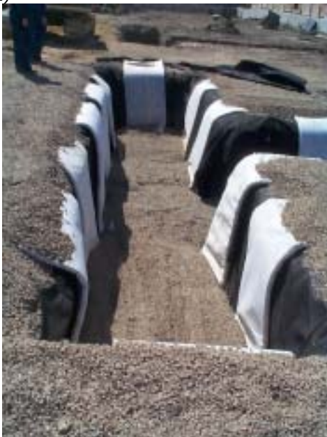
60. Construction of gas vent layer in trench in east section of site (14/11/02)
