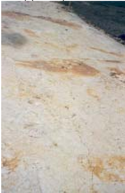
21. Minor surface cracking in finished clay cap (cracks surficial only) (31/7/02)
