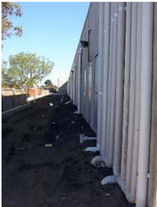
80. Gas vents stacks (4/9/03)
