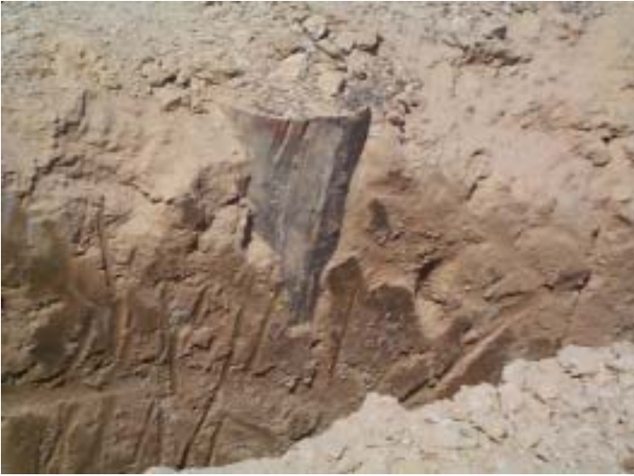
56. Pile adjacent to service trench (note limited depth of any cracking or gap around pile) (14/11/02)
