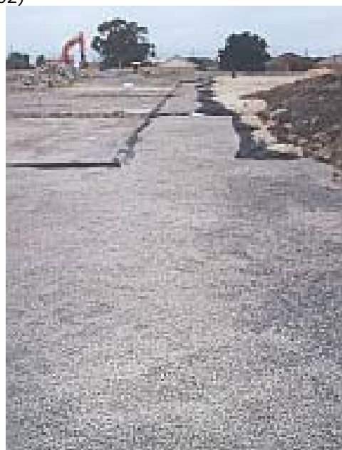
65. Construction of gas vent layer and clay cap on east section of the site (14/11/02)
