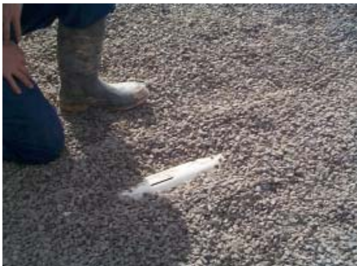
30. Horizontal gas collectors in gas vent layer beneath super market (20/8/02)
