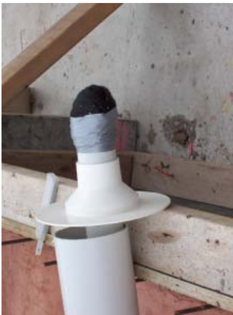
74. Bottom of gas vent assembly (17/6/03)
