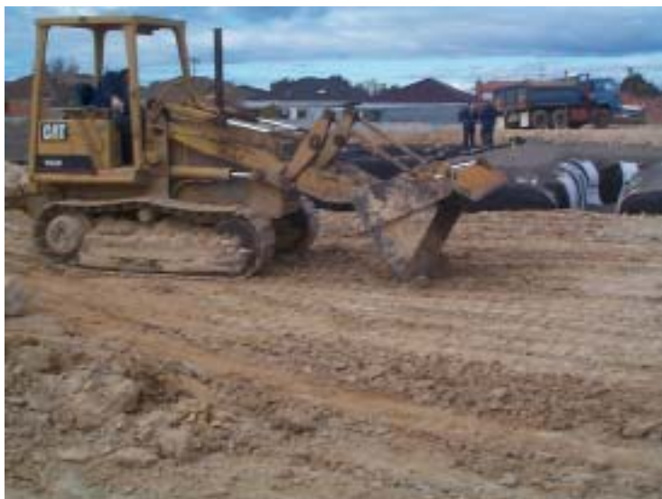
34. Scarifying surface of compacted clay layer prior to placement of next lift of clay (20/8/02)
