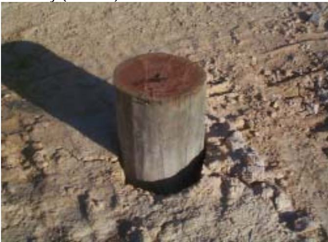
43. Typical pile showing gap and cracking near surface (25/9/02)
